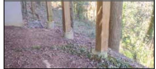
BEFORE: Concrete footings settled as retaining wall failed
