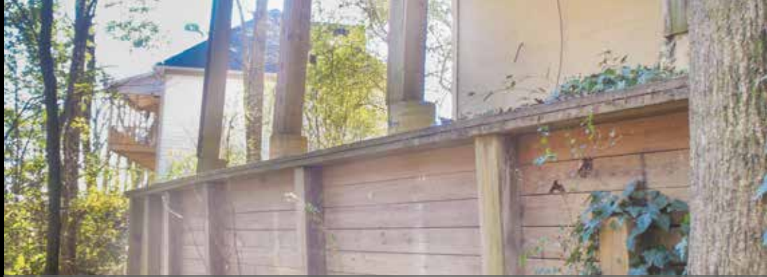
BEFORE: Retaining wall failing
