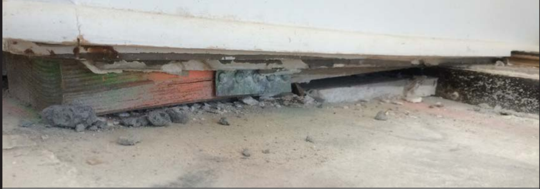
BEFORE: Foundation settlement caused floor separation
