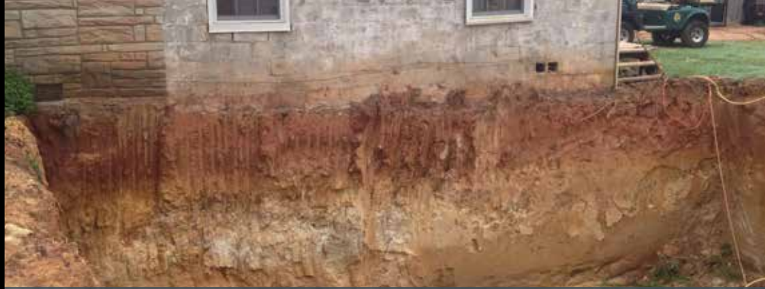
BEFORE: Unsupported foundation
