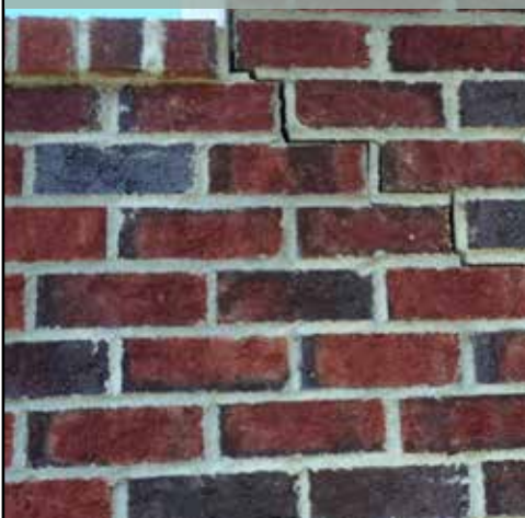
BEFORE: Crack in exterior brick
