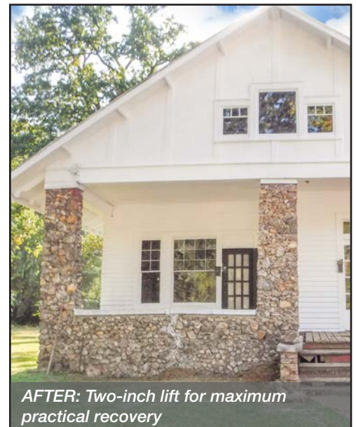
BEFORE: Porch and column settlement
